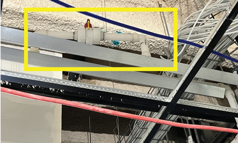
PVDF system (highlighted in yellow box) installed in plenum. Photo courtesy of MTech Mechanical
